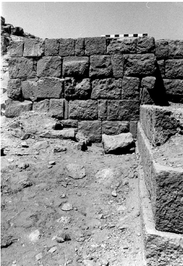
41c. 2091: eastern facade of the eastern extension, probably a blocked southern doorway. (The upper course, left of the photo scale, is restored.) That this extension was built against 2089 before it was reduced in height is demonstrated by the awkward way its right corner is supported where one of the stepped facade blocks has been removed. The contrast between the rough finish of the blocks in the central area, where the doorway would have been, and the smoother blocks to the left is also suggestive (rg 10-17, 1989)
