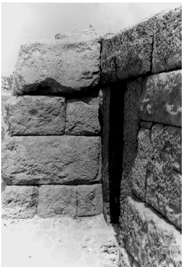
119a. 2230+2231: detail of southern doorway. Left of the far jamb is the angled scar made by the abutment of the battered wall of 2231 during Phase ii, when the entrance was at the north end of the corridor (amr, 1990)
